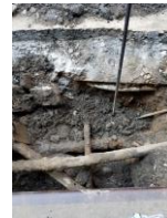
Electric and wastewater infrastructure, NYC
